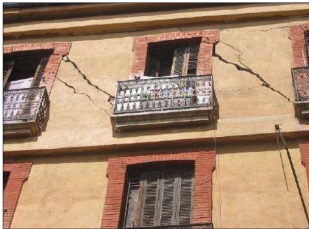
Photo 1. Badly damaged facade in Belouizdad
